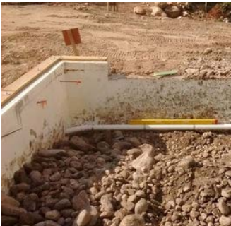
Septic-System Drainpipe Runs Through the Garage ... Huh?
